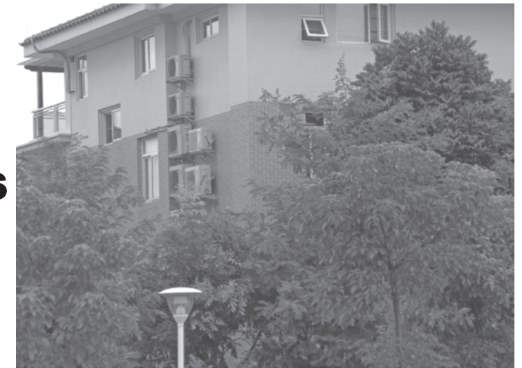
Split type air conditioner and window type air conditioner. Installed on exterior wall-big exposure.
