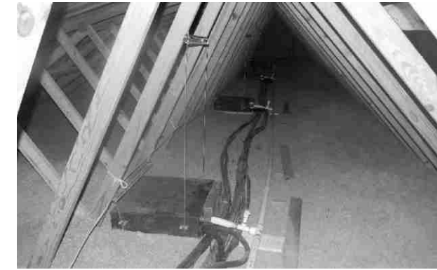
Mounting-Threaded Rod Hung on Truss
